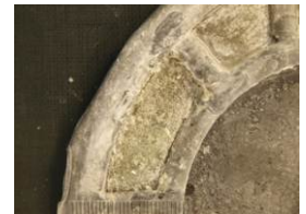
6. Dry, flakes of coating remain
